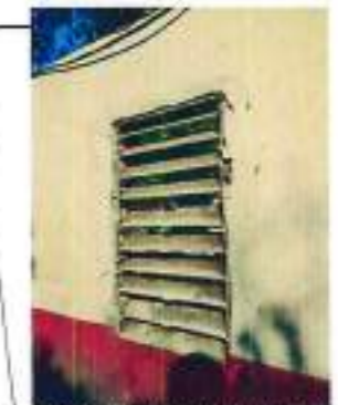
EXISTING LOUVER WINDOW TO BE REMOVED AND FILLED WITH CONCRETE, CEMENT PLASTER AND PAINT FINISH (COLOR: TO ARCHITECT'S APPROVAL)
